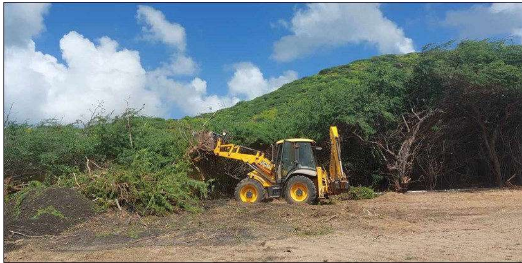
Figure 17: Machinery is used to clear Mexican thorn along road verges © L. Shearer
